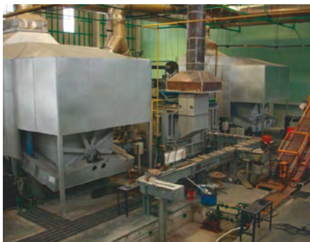
A 15 tonne holding furnace recently commissioned in Thailand
