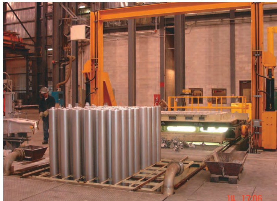
One of the very impressive items of plant central to the operation of Matalco’s 90,000-tonne-per-year recycling plant was this Mechatherm vertical 30 tonne D.C. billet casting machine
