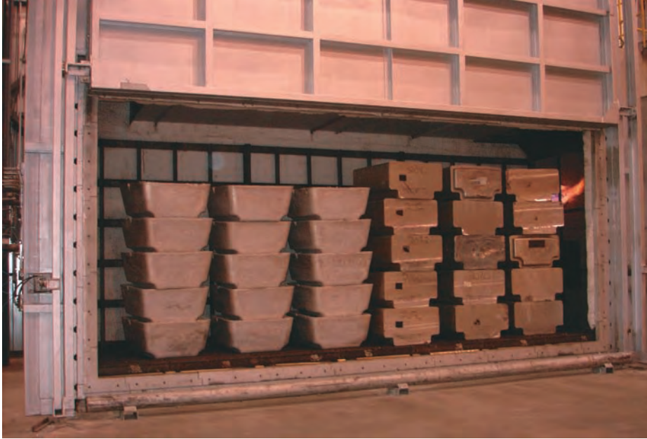
The Mechatherm solid scrap preheating oven installed as part of the major project at Metalco, Canada
