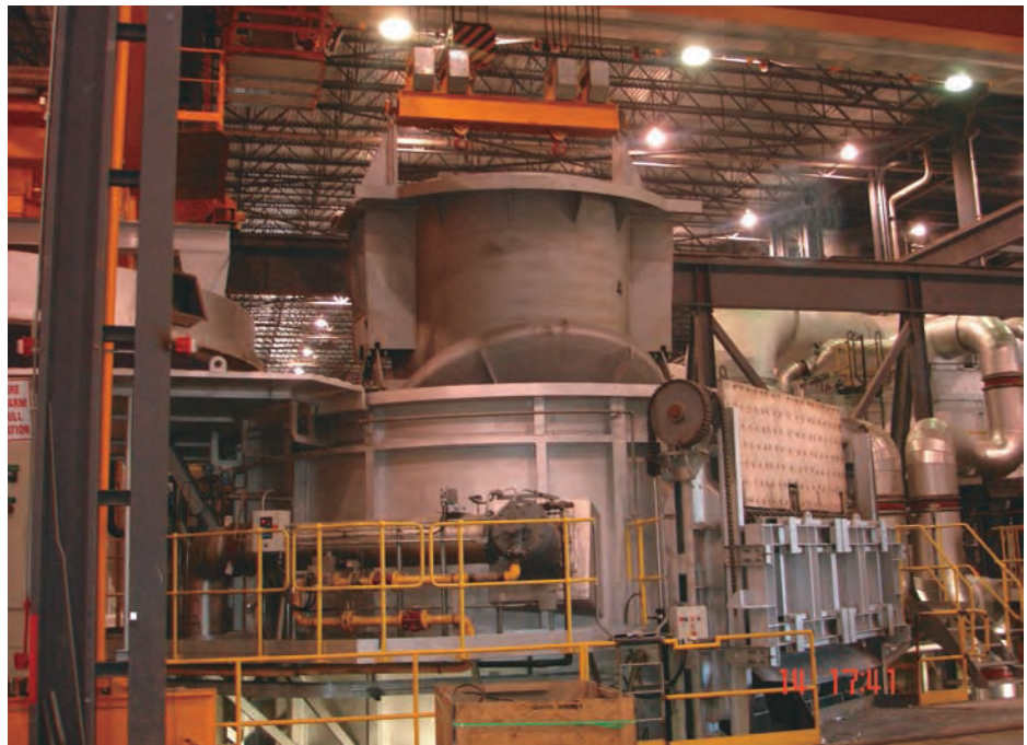
Another essential part of the Metalco contract were these Mechatherm 32 tonne melting furnaces, both equipped with charging buckets
