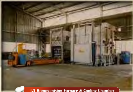
12t Homogenising Furnace & Cooling Chamber
