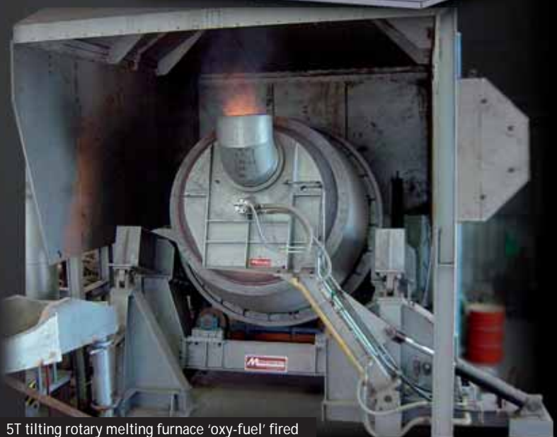
5T tilting rotary melting furnace 'oxy-fuel' fired
