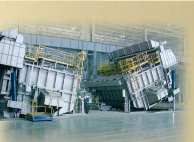
2 x 60T Electrically Heated Tilting Holding Furnaces Feeding Two Continuous Ingot Casting Machines
