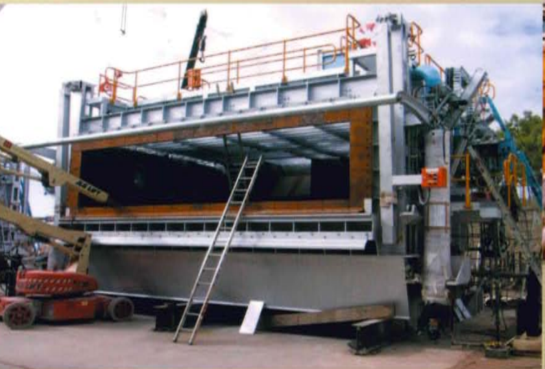
55T Tilting Holding Furnace Pre-assembled Ready For Transportation to Site
