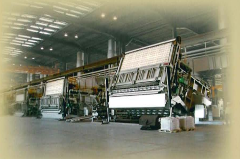
4 x 45T Gas Fired Tilting Holding Furnaces Feeding Two Continuous Casting Machines
