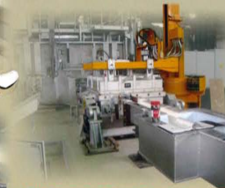
SNIF Degassing Unit and Ceramic Foam Filter installed by Mechatherm
